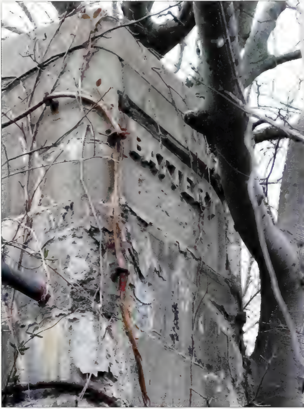
Figure 3.9. View looking northeast at corner of structure, Battery Peck. Efflorescence can be seen on many of the vertical surfaces and spalling is present on both horizontal and vertical surfaces indicating water has penetrated the concrete and is damaging the material (Olmsted Center, January 2009).
